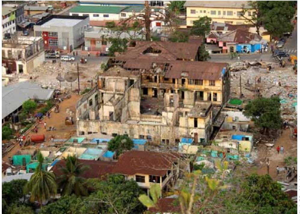
Prior to its demolition in April 2012, Old Government Hospital had been home to settlers and their families for over 20 years.
